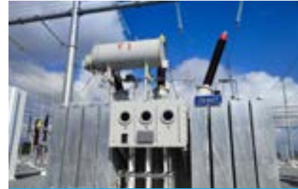
Johor Yondr Datacenter 275kV 90MVA Transformer
