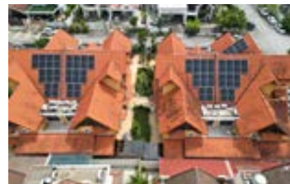
Kuala Lumpur 42.9kWp Solar PV Residential Project
