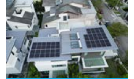
Subang Jaya, Selangor 14.3kWp Solar PV Residential Project
