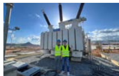
Luzon Aboitiz Power 75MW 230kV Bugallon Substation for Solar Project
